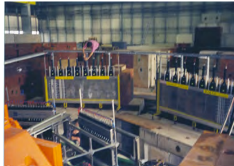
Figure 2. Mounting Preshower Detector at CERN – East Hall
